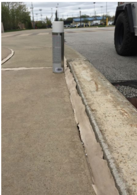
Picture 4: Level Changes at Curb-to-Sidewalk
