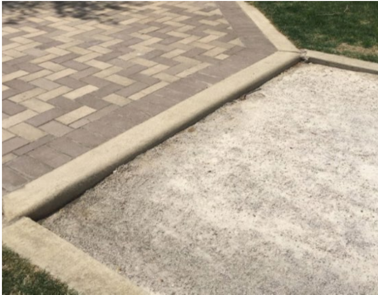
Picture 3: Level Changes at Dissimilar Materials
