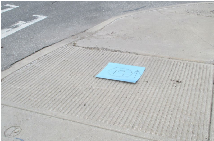
Picture 5: Deteriorated Sidewalks
